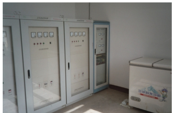
Figure 5: Cabinets with inverters and AC-distribution. Typical chest freezer to the right
