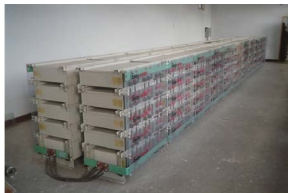
Figure 4: Battery bank in the power house, AGM type, lead acid
