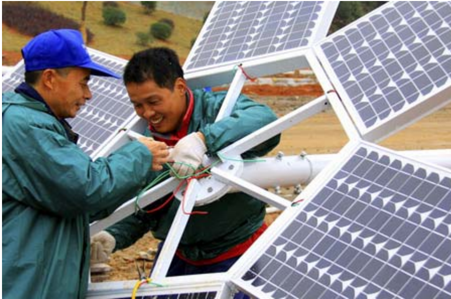
Technicians assemble a solar-powered street lamp in Jing'an county of Jiangxi province on December 11. Official statistics showed China as a leader in hydro and solar power usage last year. [China Daily]
