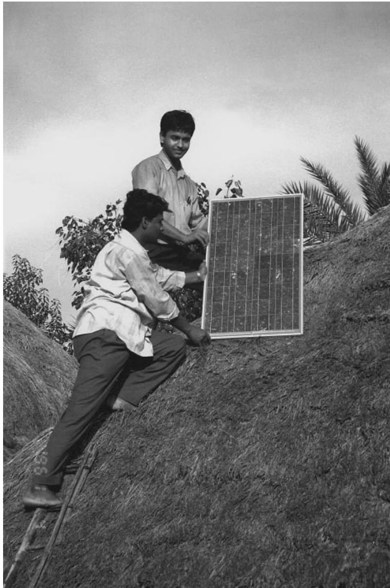
Figure 2. Ramakrishna Mission installation team mounts the PV module to the thatched roof of a village home. (Credit: NREL PIX 04875)
