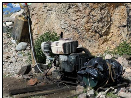
A typical gasoline-powered generator used to provide electricity in rural areas.
