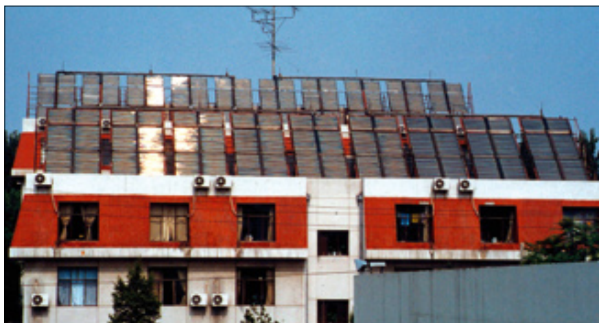
Practical test: Installed in 1989, this is the first system with Al-N/Al tube collectors to be installed outside the university.
