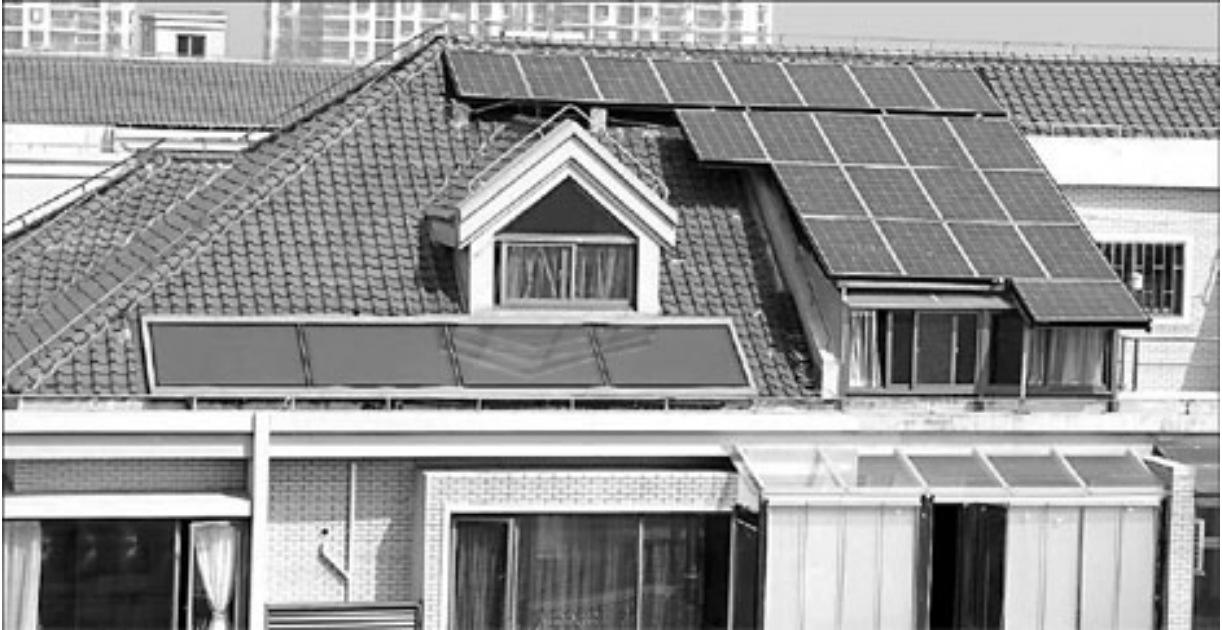
The roof of Zhao Chunjiang's apartment in Shanghai is covered by 22 solar panels.
